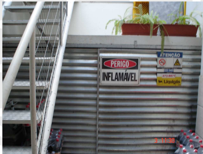
Picture: Gas cylinders stored on the premises (hazard risk).
